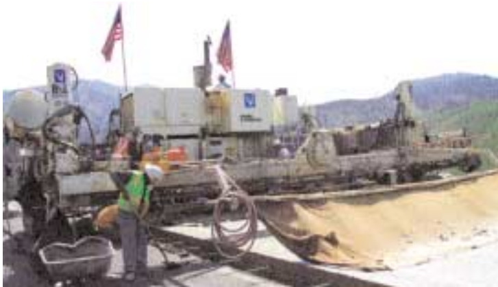
Inserting tie bars on the first of four paving passes, slipping a lane and shoulder on the outside.
