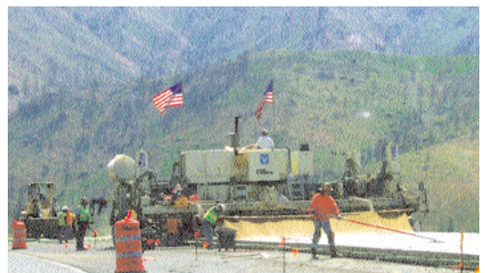
Paving a five-mile stretch on I-80 in the Sierra, just east of Truckee.
