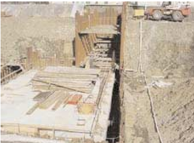
Pump plant and storage box
