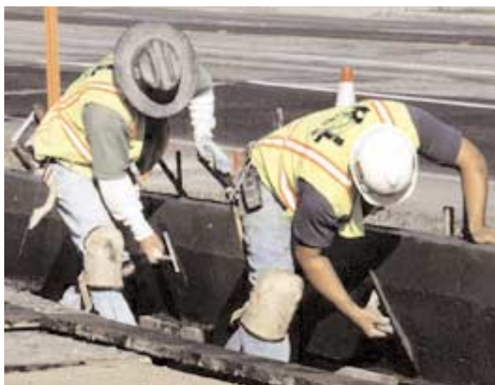
Construction of concrete header. The barrier that separates train tracks and roadway.
