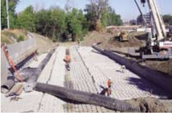
Concrete cellular mats at Santa Clara inlet.
