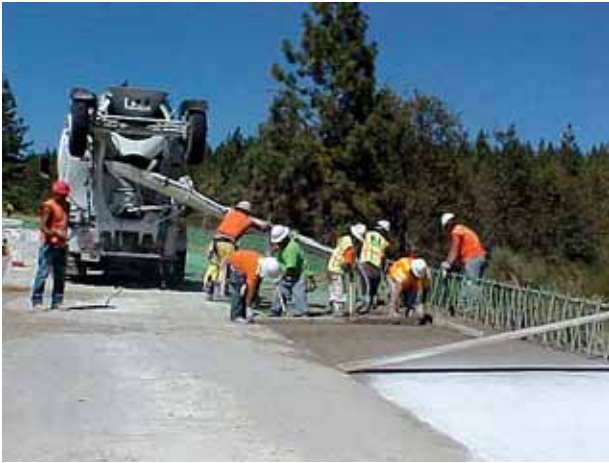
The existing roadway was bounded on both sides with asphalt shoulders. The contract called for shoulder-to-shoulder concrete pavement rehabilitation.
