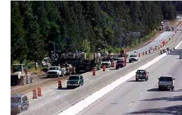
Work was done in very tight quarters. Some traffic came down the hill at 70-80 miles per hour. Three CHP officers directed traffic.
